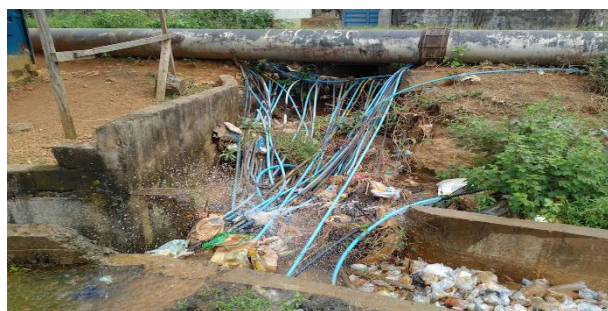
Figure 5: Leaking ‘spaghetti’ lines connected to a water main in Freetown (credit: ASI)
